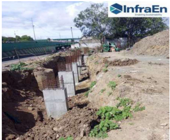
4 pre cast column beam reinforcement ready for fixing, Sathy road transfer station
